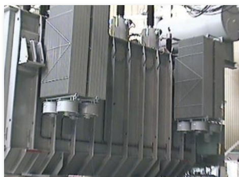
▼ Heat generation in a 225 MVA transformer: the coolers are still shut
