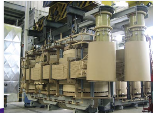
▼ The interior of a 225 MVA transformer: reels and cables are covered with cardboard
